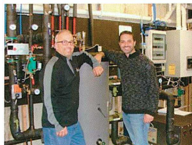
The Mechanical Room at 25 Orchard Lane
